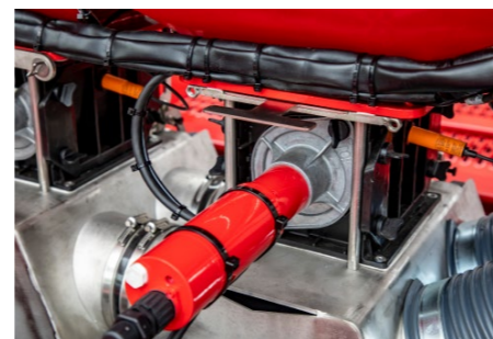
Metering unit – pressurised hopper system with valve
